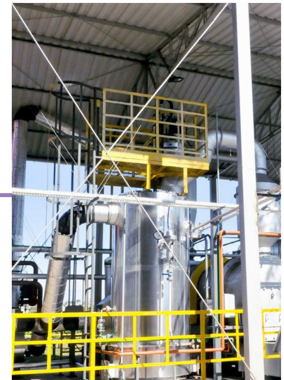
Barueri STP's plasma gasification equipment, in the SPMR
