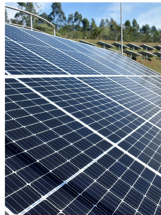
Sewage treatment plant in Mogi Mirim with a photovoltaic power generation system, installed in partnership with SESAMM (Mogi Mirim Sanitation Services)
