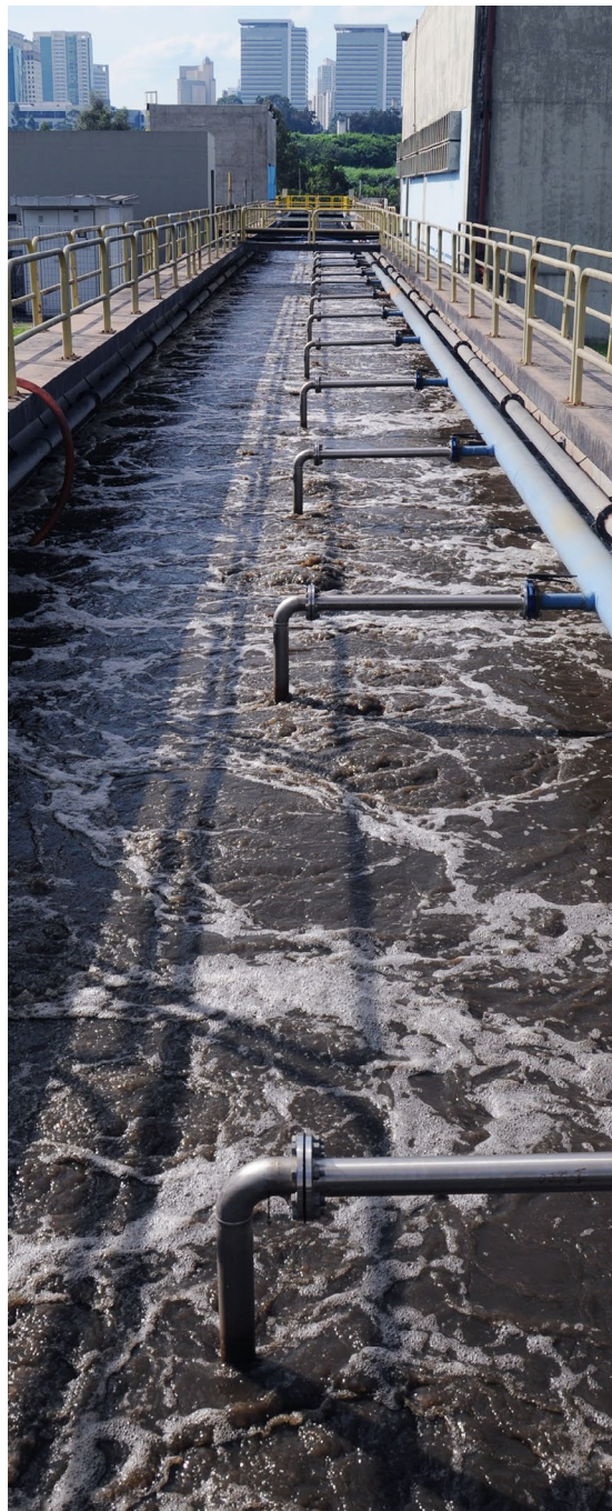
Tank of the Company's largest sewage treatment plant, ETE Barueri, in the west of Greater São Paulo
